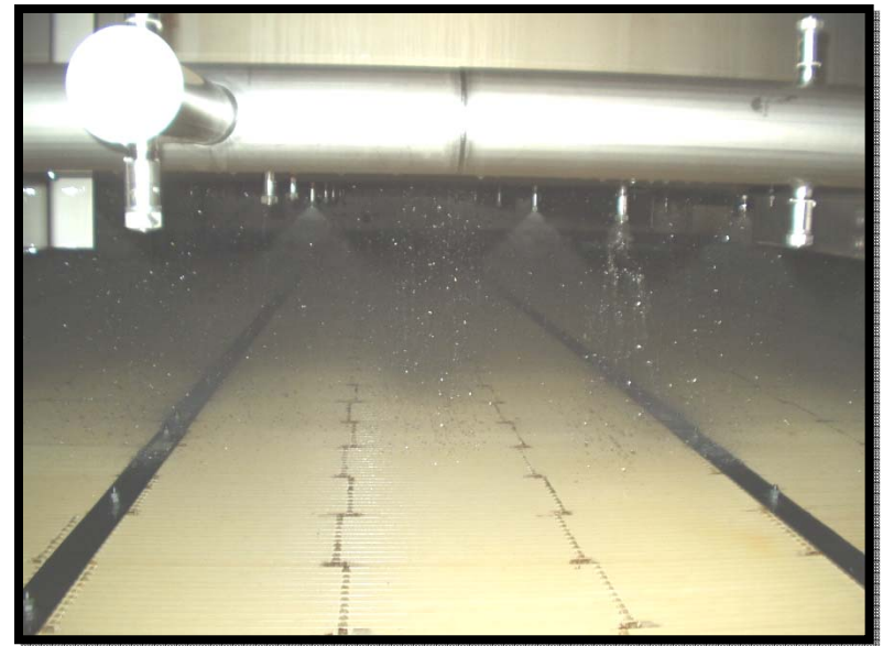
Mist Eliminator Wash System
